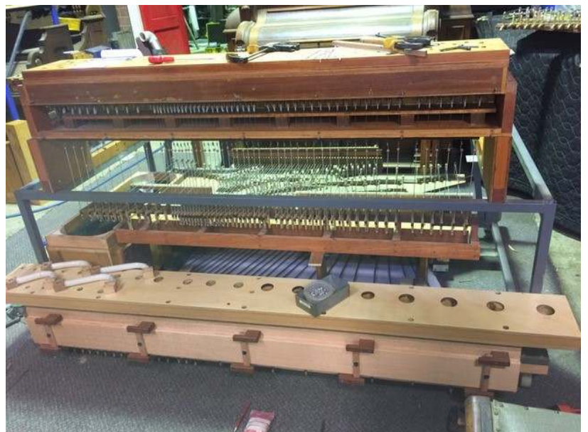
New Pedal chest installed at the rear of the organ with Swell action installed
